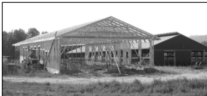
Parlor under construction at Wilson Farms, Dansville, NY. The contractor had a complete set of plans with all major decisions made before preceeding with construction.
