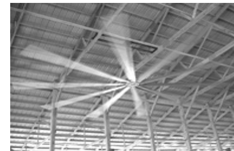
Figure 2 Position of large HVLS overhead fan in a freestall barn.
